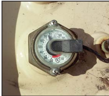
Propane Tank Gauge
